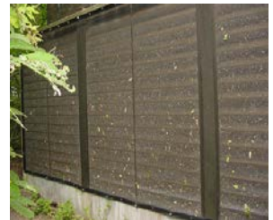
Air Intake Louvers
