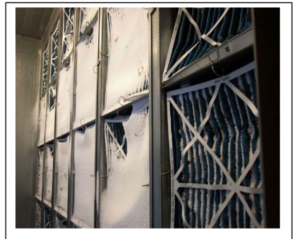
Snow shown building-up and damaging pre-filters
