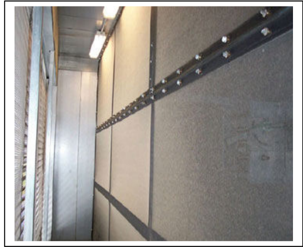
Air Intake Filters Stopping Cottonwood Seed from Reaching Pre-Filters
