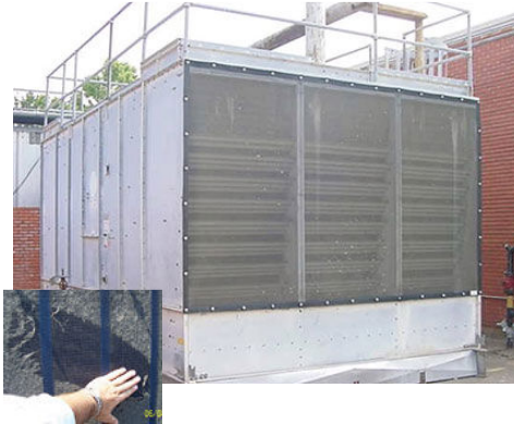
Cross Flow Cooling Tower
