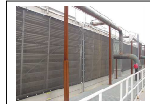
Air Intake Filters Protecting a Process Cooling Tower
