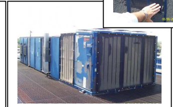
Air Intake Filters Protecting Chiller Coils from Cottonwood Seed
