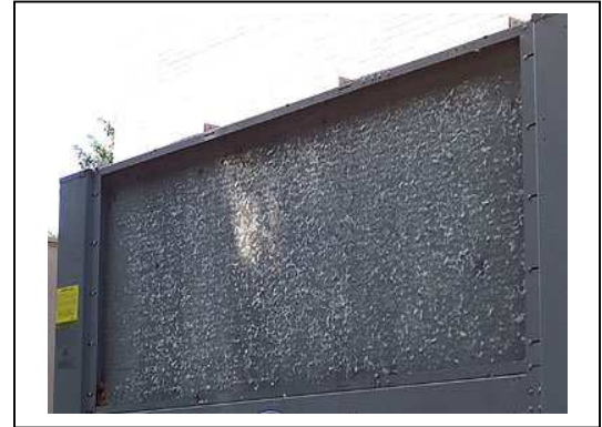
Coils Severely Fouled With Cottonwood Seed
