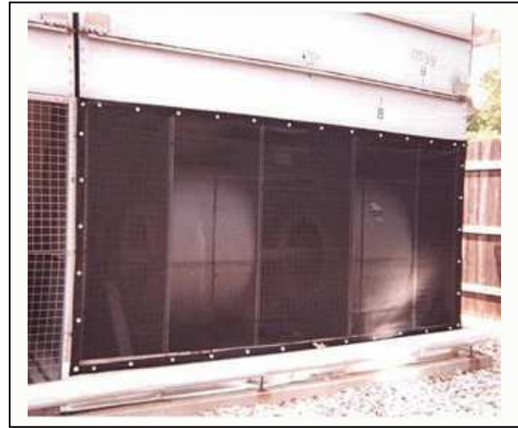
Air Intake Filter On BAC Cooling Tower
