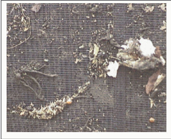
This Is The Kind Of Debris That Will Clog Cooling Tower Strainers & Heat Exchangers
