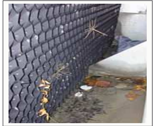
Debris & Sludge Build-up in Cooling Tower Sump
