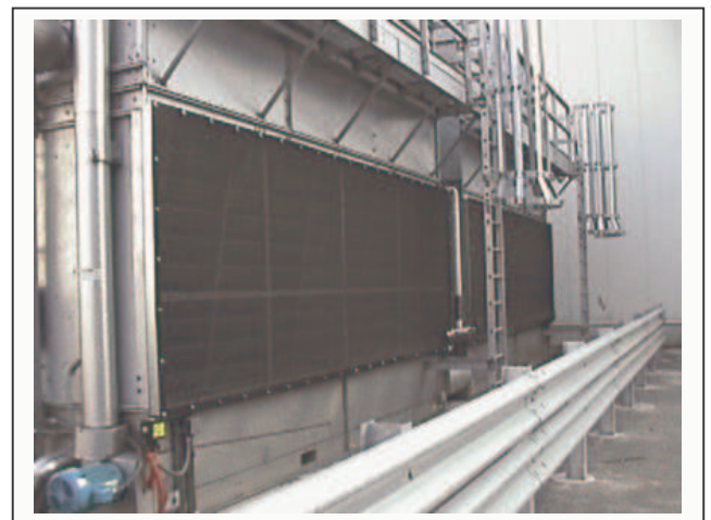
Air Intake Filter Keeps Airborne Debris Out of Cooling Tower
